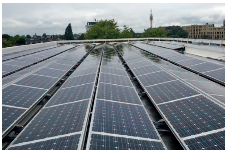
Pv-panelen energieneutrale school
